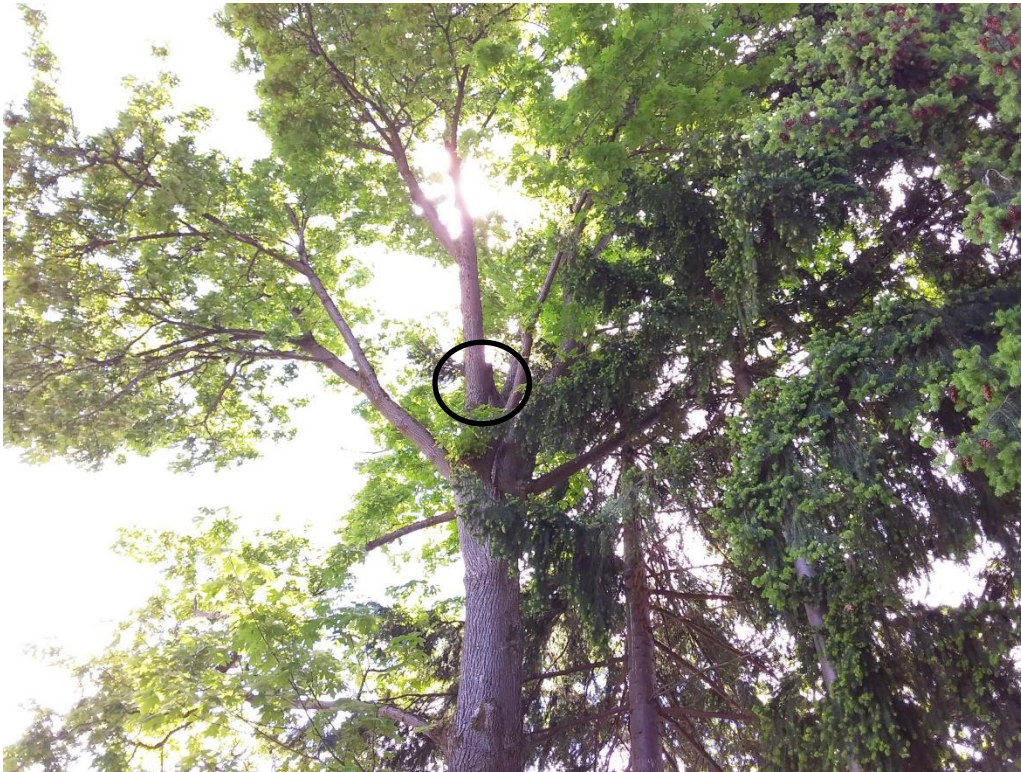
Figure 26. Looking up into the canopy of the #13 tree. The large breakout point is just visible (circled).
