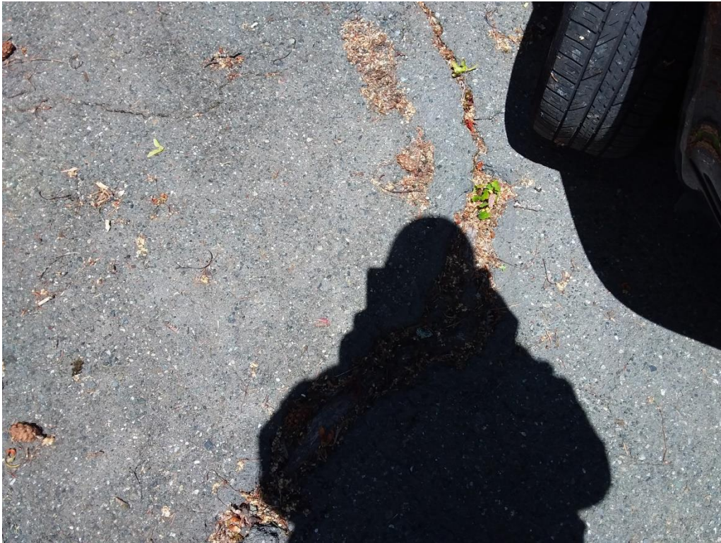
Figure 27. Uplift in the asphalt from the #13 maple roots.
